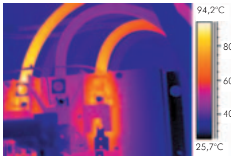
See loose connections
